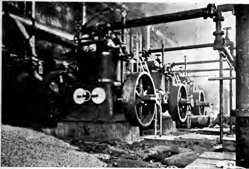
FIG. 5.—PUMPS FOR CONDENSER INJECTION WATER.
